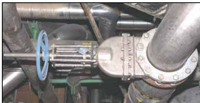
Post refiner line isolation.
